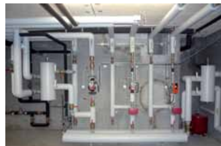
District heating substation, Grenoble, Frankrig.
