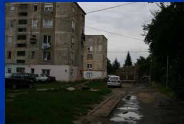
Degradation of blocks' facades
