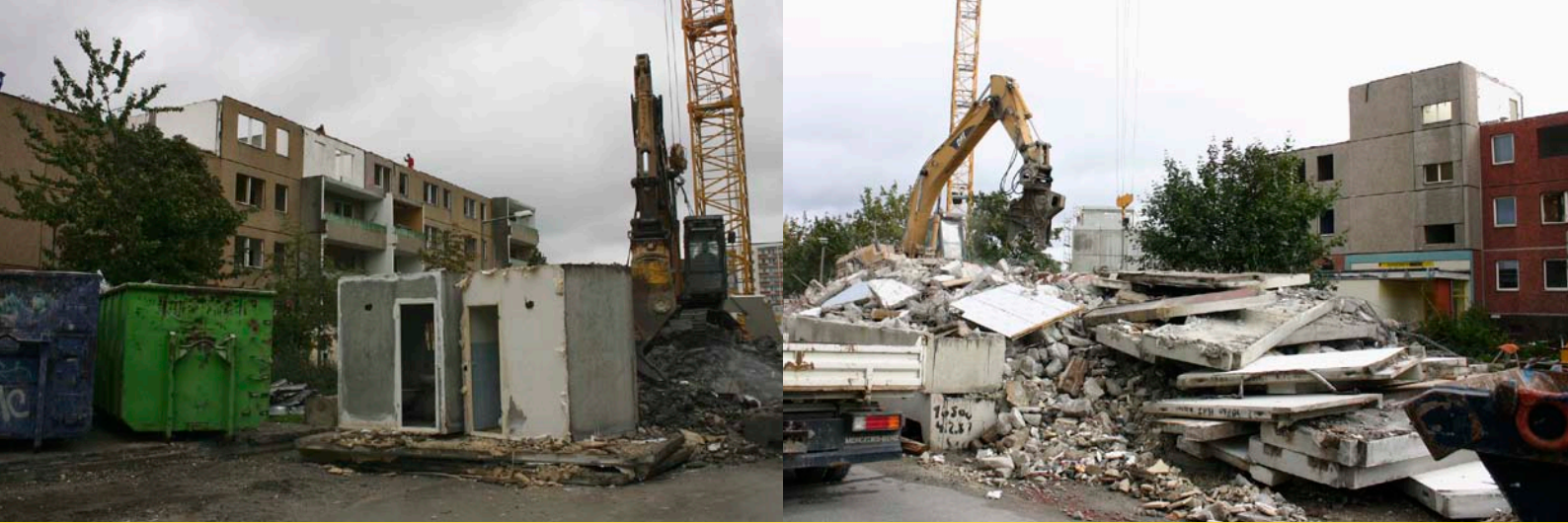
7-8. DEMOLITION OF BUILDINGS IN MARZAHN, ONE OF THE PREFABRICATED HOUSING ESTATES IN BERLIN
